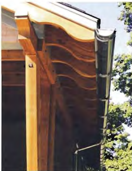
The eaves that CK Architects added use natural wood — in this case Douglas cut to a decorative outline — and raw aluminum gutters to counterpoint the painted trim and siding.
